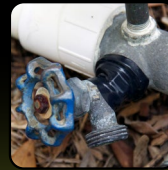
Repairs loose or leaky plumbing
